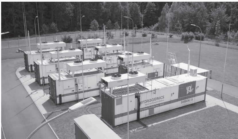
Power-to-Gas Pilotanlage © Uniper
